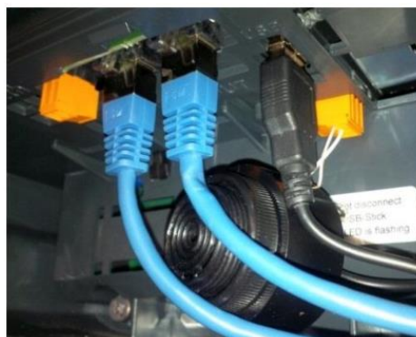
Figure 6. Buzzer connection with Signal relay and 5V USB power supply
