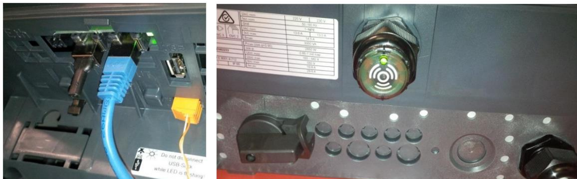
Figure 5: Signal Relay using 12Vdc supply from RJ45 (left) with 12Vdc buzzer mounted to underside of inverter (right)
